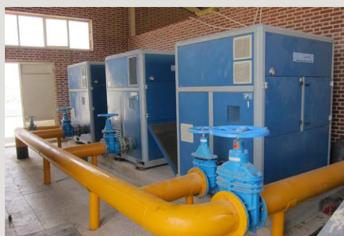
Blower station at Moorche Khort.
