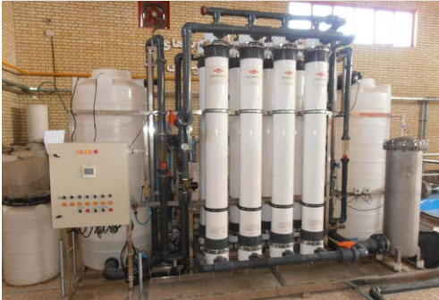
Ultrafiltration Plant in the Morcheh Khort WWTP.
