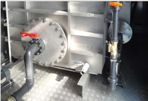
The pilot plant for innovative wastewater technology was put into operation in 2014.
