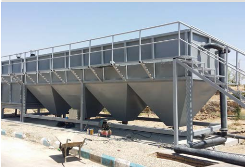
Chemical Sedimentation - Morcheh Khort Wastewater Reuse Plant.
