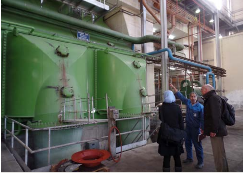
Site visit at the Isfahan Power Plant.
